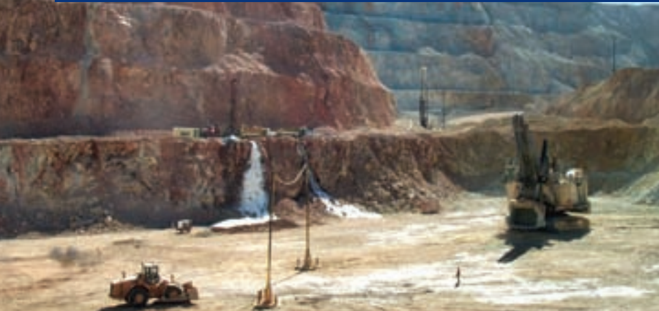
A new in-pit dewatering well at Morenci produces groundwater as it is being constructed
